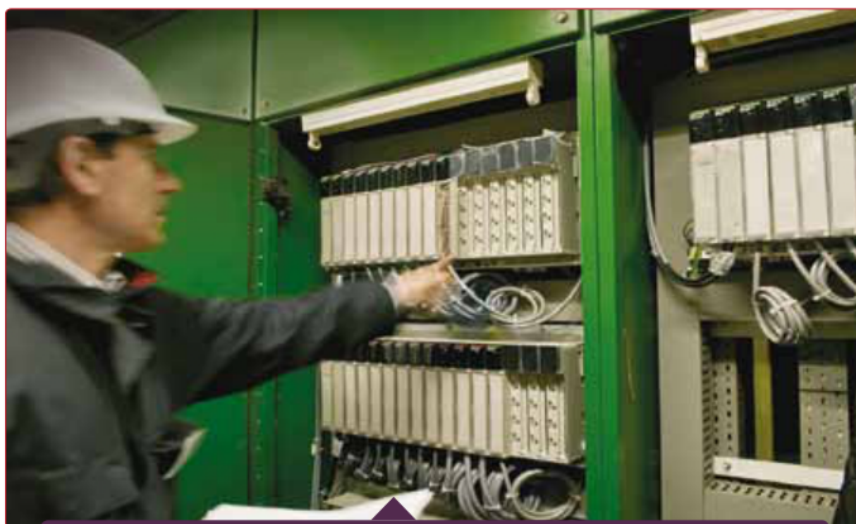
Automates programmables Schneider Electric en application.
